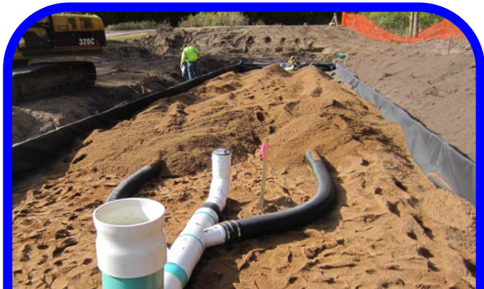
Perforated underdrains with a flow controlling valve were installed and covered with an 18 inch depth of iron enhanced sand filter material.
