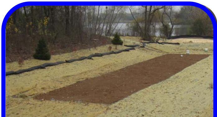
A native seed mix was covered by erosion control blanket and highlighted with shrub plantings. The cells will remain off-line until 2014 to allow the native seed to establish.
