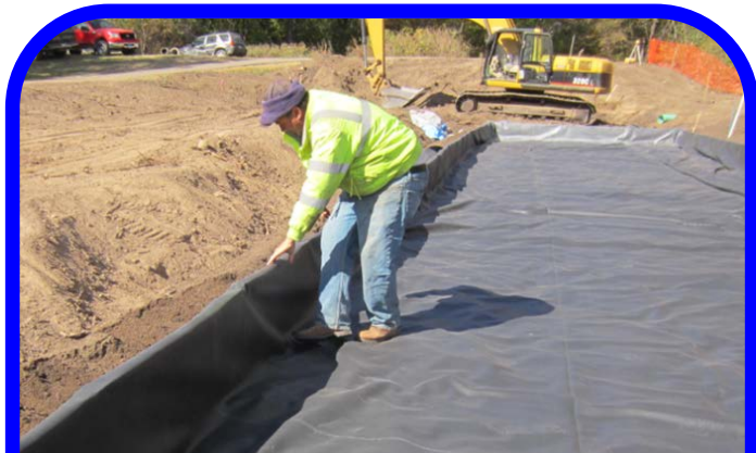
After excavating to grade, plywood forms were used to hold the rubber liner which separates the infiltration area from the filtration area.
