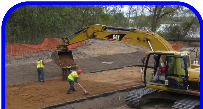
The iron sand mixture in the filtration area contained 5% iron filings by weight. The infiltration areas outside of the forms contained 70% coarse washed sand, 15% compost and 15% sphagnum peat.
